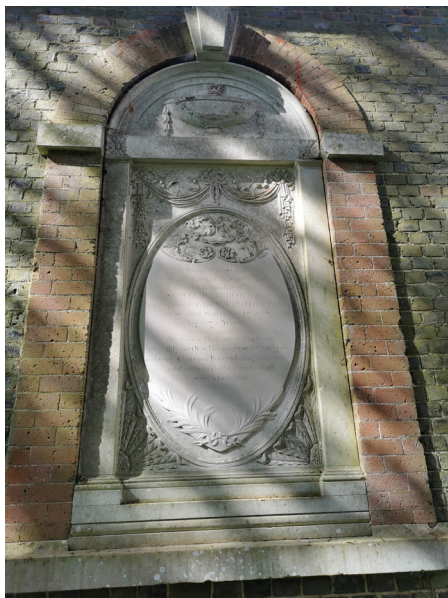
Figure 7: further repairs to the monument to Samuel Heathcote at the Heathcote mausoleum where the lettering is disappearing.
