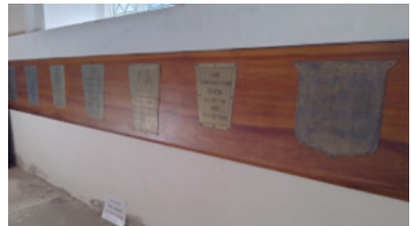
Figure 10: Coffin plates raised after vandalism in the vault. Photo E. Blood
