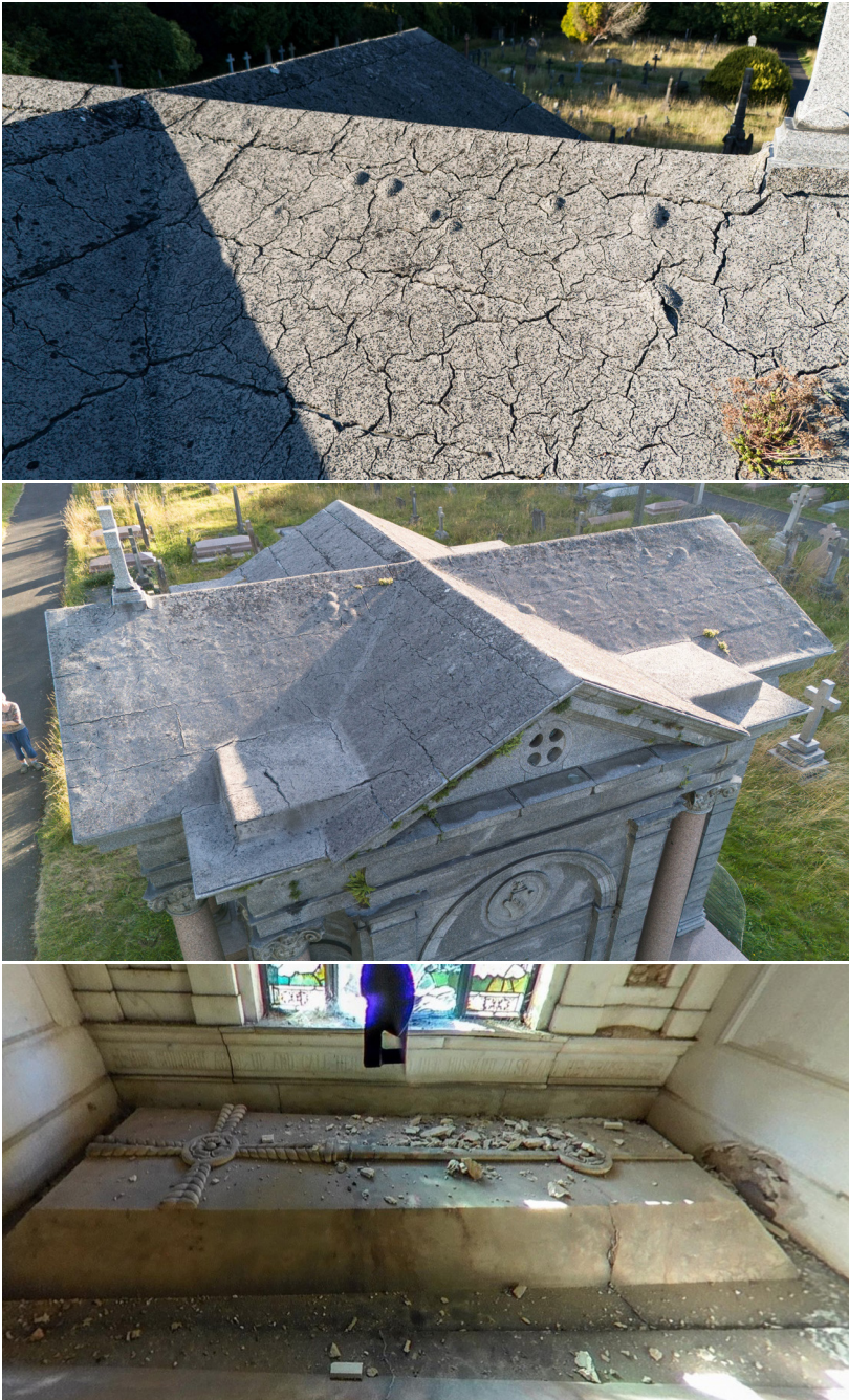
Figures 3, 4 & 5: The badly cracked and bubbled bitumen roof and water-damaged interior.
